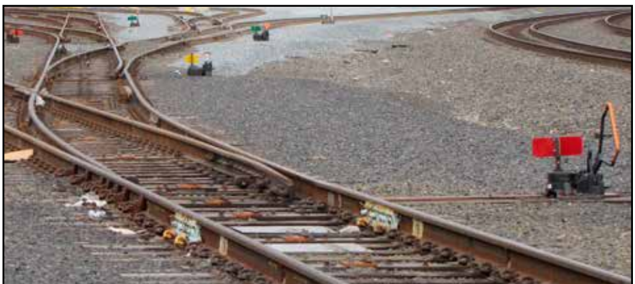
Fig. 7 Hand Throw Switch - member of train crew must get off train and manually set each switch for the desired route
