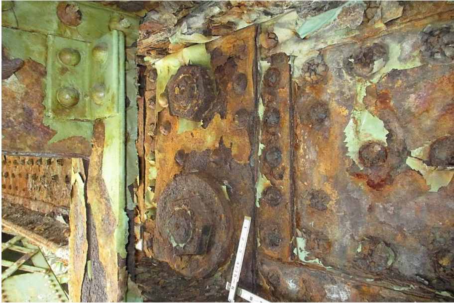
Photo 5a – Rusted and corroded pins and pin nuts.
