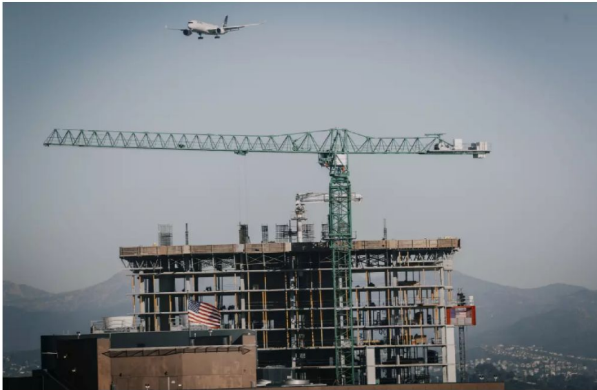
An apartment complex under construction in downtown San Diego on Jan. 16. As of last quarter, the number of new apartments under construction in San Diego County rose 10% from three years earlier, CoStar data show. (Sandy Huffaker / For The Times)
