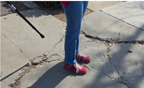
FIGURE 3. BROKEN SIDEWALKS ALONG THIRD AVENUE MADE TRAVERSING DIFFICULT FOR THOSE USING MOBILITY AIDS.
