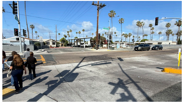
Figure 4. An intersection on Naples Street and Industrial Boulevard with unmarked and faded crosswalks along with signal malfunction.
