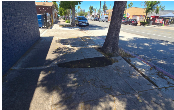
Figure 3: Uneven and broken sidewalks observed all throughout Imperial Avenue.
