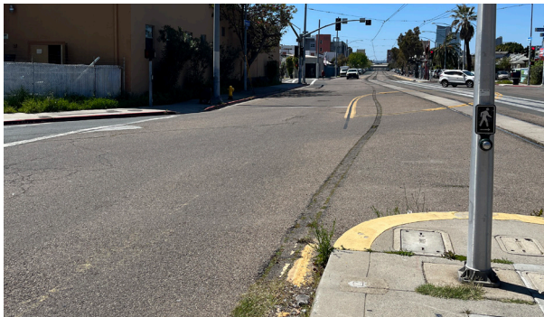
FIGURE 3: MISSING CROSSWALK IN THE INTERSECTION OF COMMERCIAL STREET AND HARRISON AVENUE
