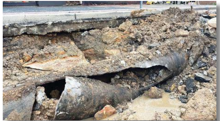
Burst main on Willoughby Rd
