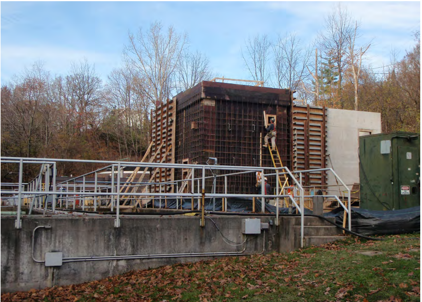
Waterdown Wastewater Treatment Plant. PHOTO City of Hamilton
