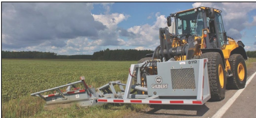
Brush mowing is a viable alternative for roadside vegetation management | Photo: Gilbert
