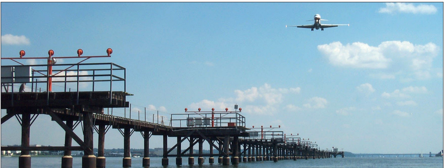
Runway approach lighting at Runway 1 at Ronald Reagan Washington National Airport. At 2,094 meters in length Runway 1 has an approach lighting structure out into the water to a distance of 820 meters from the threshold.
